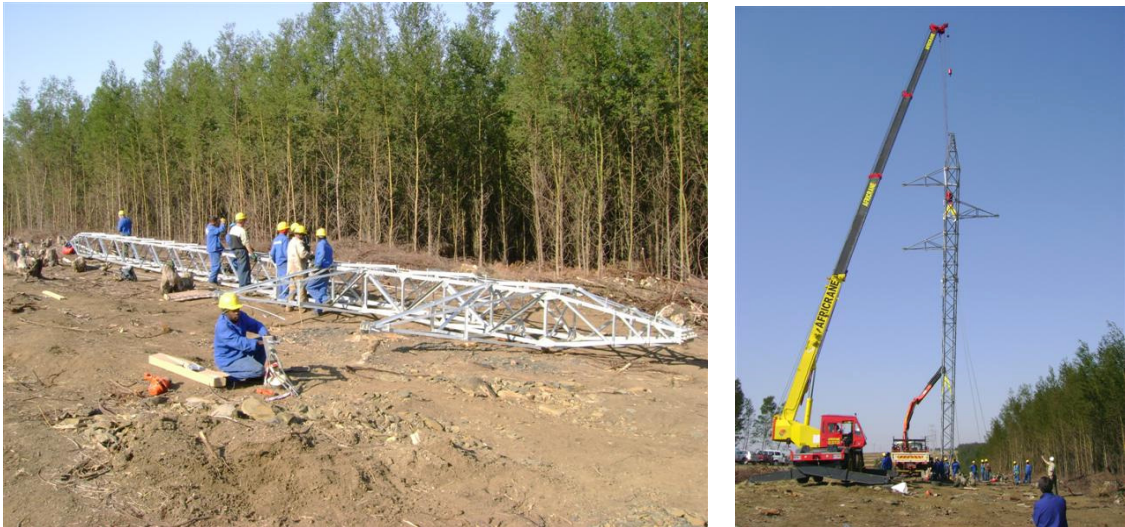
Figure 11.6-2: A guyed structure being assembled on its side (left) and hoisted, once assemble, into position by a crane (right). The crane would hold the structure in place until all four stays are secured.
