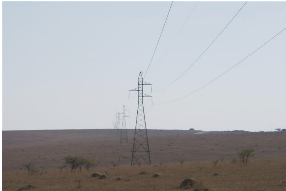
Figure 11.1-1: An 88kV power line in Zululand
