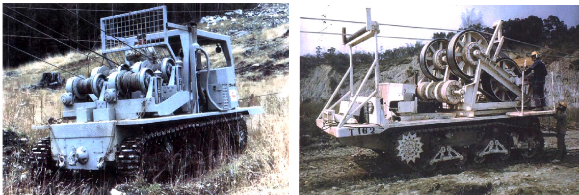
Figure 11.6-5: A winch (left) and tensioner (right) in operation during the stringing of an overhead power line. (Morcap Industries 2008)
