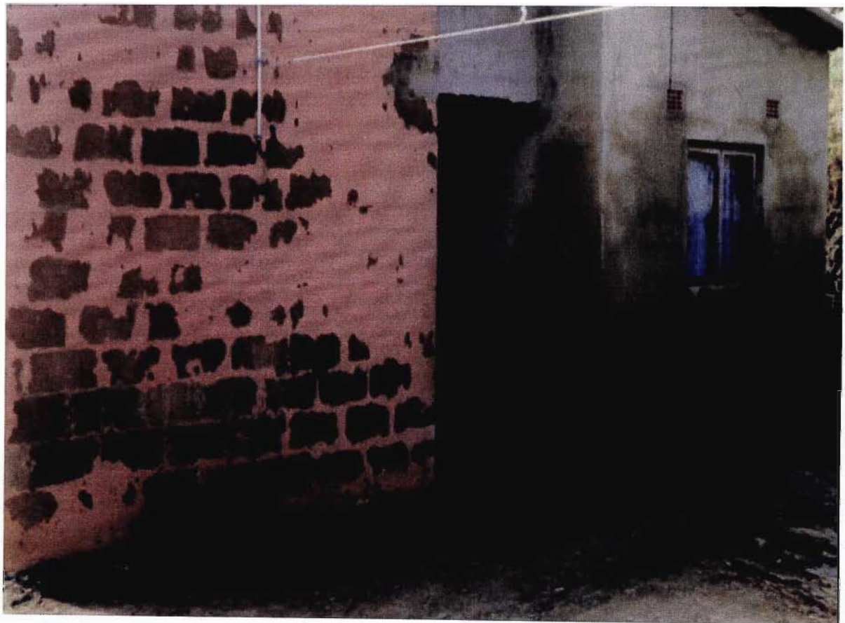
FIGURE 6 : Wall covering of walls that were painted only (left) and plastered only (right), and the effects of dampness.
