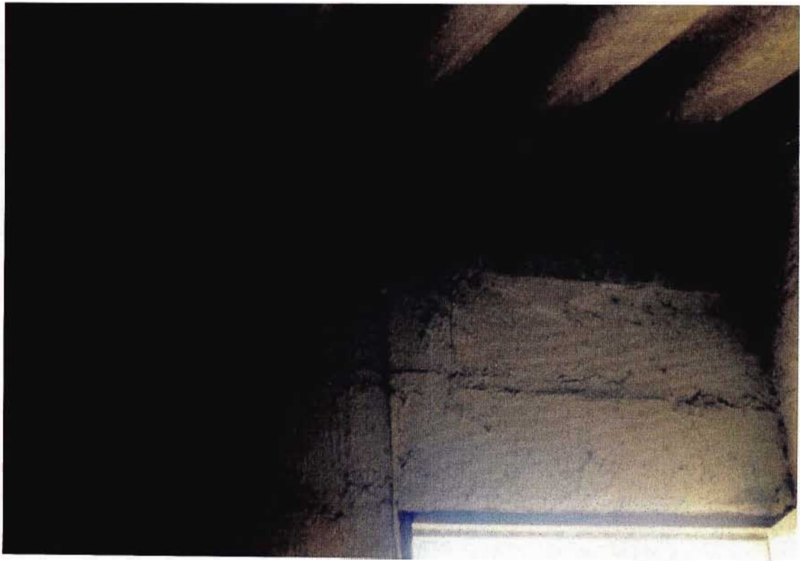
FIGURE 7: Interior of a dwelling indicating the absence of airbricks, and an asbestos roof which also serves as a ceiling.
