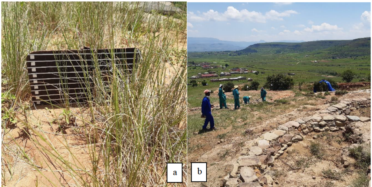
Plate 1.1: Splash plate (a) installed on-site to measure the splash erosion after storm events. Results are recorded by the community and (b) the community installs stone packs to prevent further expansion of the existing gully network.
