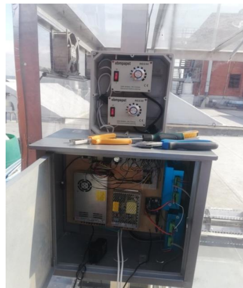
Figure 3-7: Electrical control boxes.
