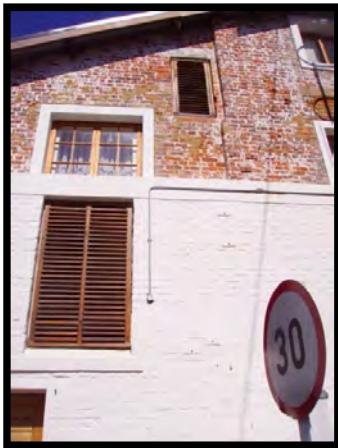
Figure 15 - The exposed brickwork adds to the tangible history of the structure, yet it is paired with modern fixtures and fittings to bring the building up-to-date. SOURCE: image taken by author
