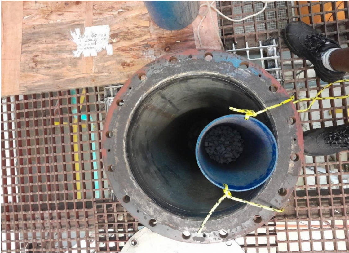
Figure 3-16: Non-Uniform Packing Arrangement (Small packing at the side)- During Vessel Loading
