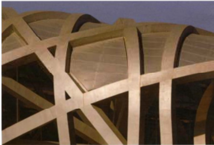
Figure 38. Solid and void effect by the roof membrane and the solid appearance of the steel framework. (Brown, 2009:36)
