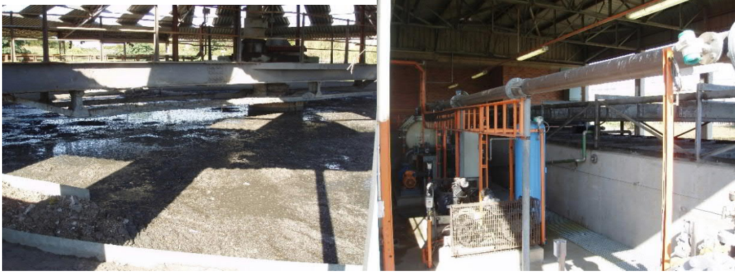
Figure 4-4 KwaMashu WWTW (2020) - Left: Gravity Thickening Unit, Right: DAF Thickening Unit
