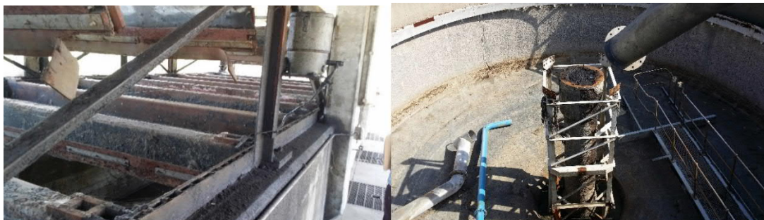
Figure 4-3 Northern WWTW (2020) - Left: DAF Thickening Unit, Right: Gravity Thickening Unit
