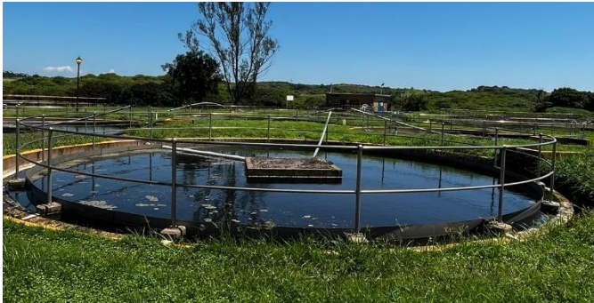
Figure 61. Clarifier Tank (Author, 2023)
