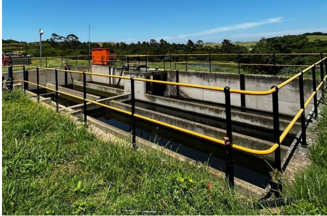
Figure 65. Final Effluent Tank (Author, 2023)
