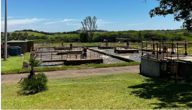
Figure 62. Aeration Tanks (Author, 2023)
