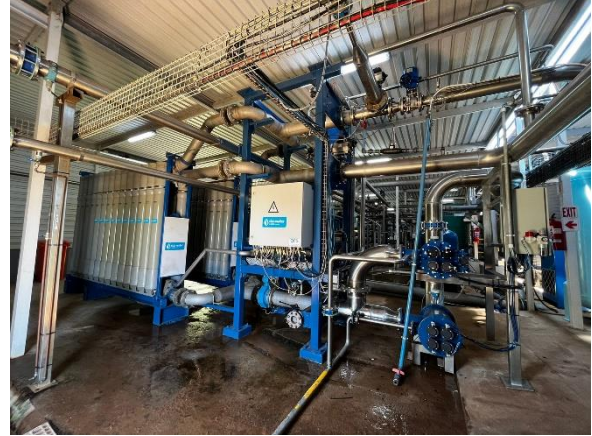
Figure 66. Inside the Water Re-use Plant (Author, 2023)
