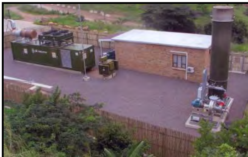
Figure 6.8 – Mariannahill landfill gas generation system (Source: Douglas, 2007)
