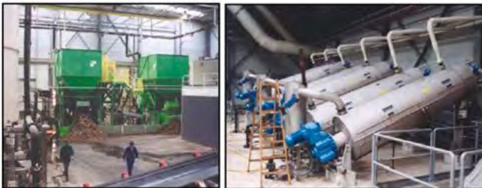
Figure 3.4 – Hydropulpers and dewatering equipment
