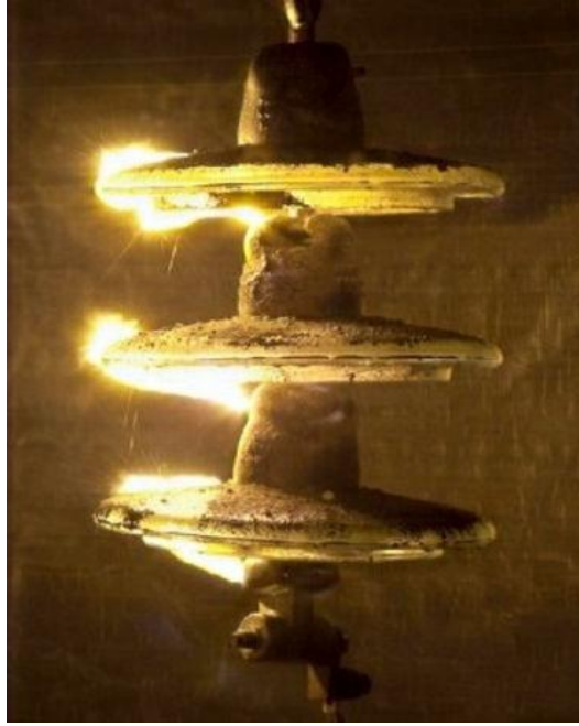
Figure 6: High voltage pollution flashover on glass cap-and-pin insulator [36].
