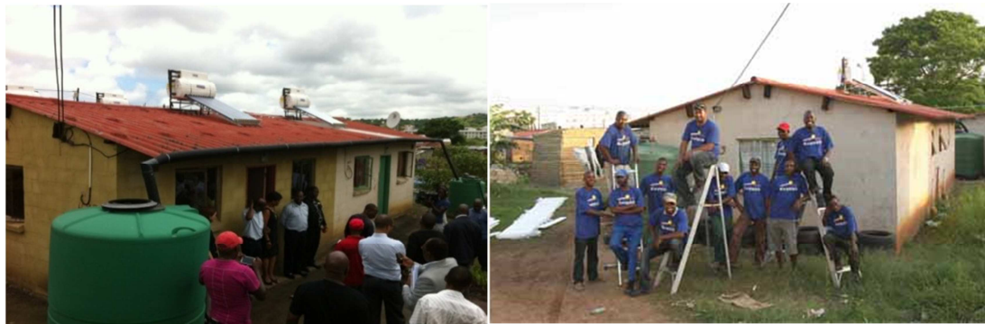
Figure 2-13: Cato Manor retrofit project in Durban. (Source: Photo from the site visit and ClimateAction, 2011)
