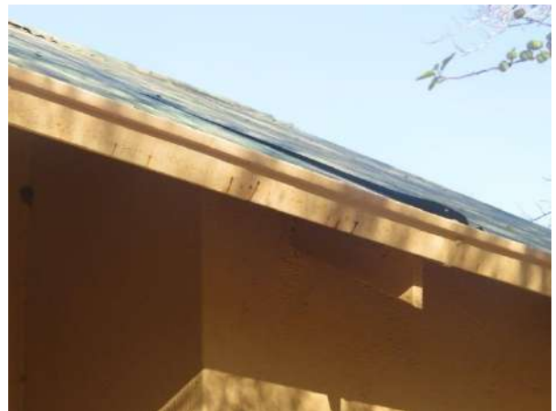
PLATE 6 2.43. Damaged Domitory roof ( Source: Author).
