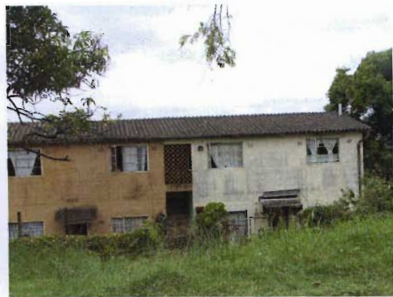
Illustration 91, Major Calvert Road flats which are in a state of disrepair and within a bleak environment
