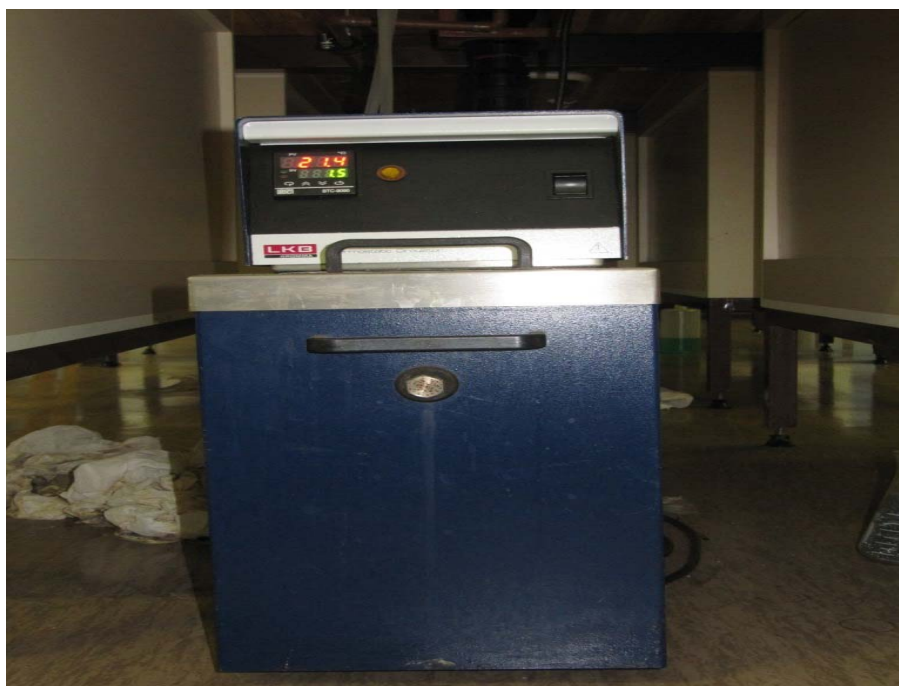
Figure A1.3 Chiller for product outlet line
