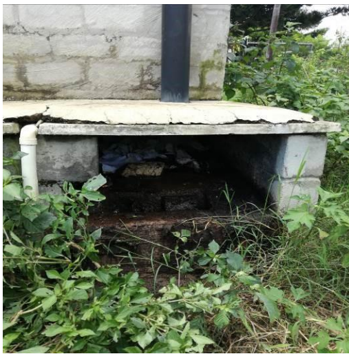
Ventilated Latrine School pits
