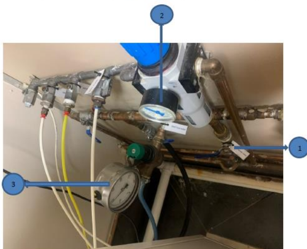
Figure 2 : Main water valve (1), compressed air gage (2) and L&W FT+ water valve (3).
