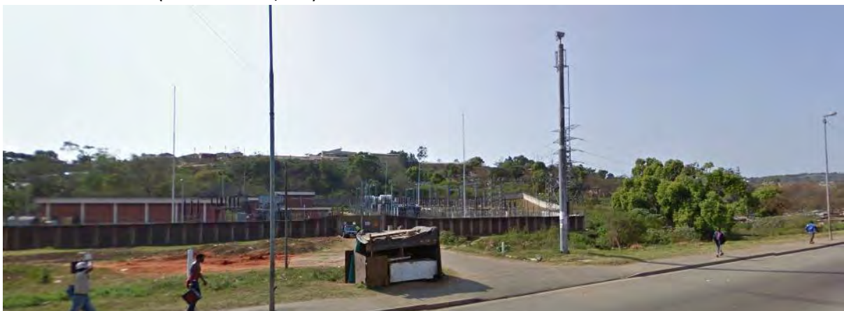
FIGURE 32: SUBSTATION (SOURCE: AUTHOR, 2014)
