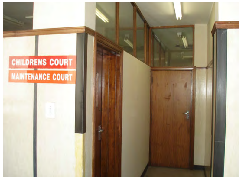
Figure 43. No differentiation between a court room door and an office (source: author).
