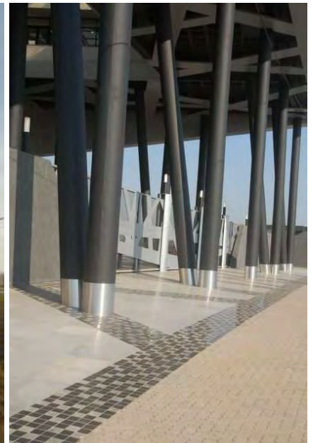
Figure 57. Tilted columns at entrance (source: DGIT Architects).
