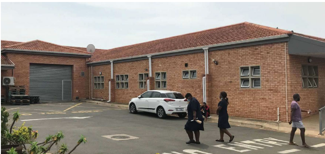
Figure 55 & 56: Eave detailing reflects a lack of considered problem solving resulting in a poor architectural aesthetic. The windows and wall on this elevation are unnecessarily exposed to high levels of solar gain, as a result of the architect not being able to manipulate the facility footprint (Author).
