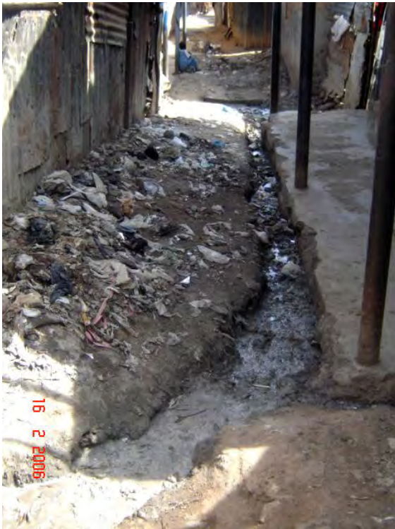
Photo 8. 15 Gabage along drainage channel
