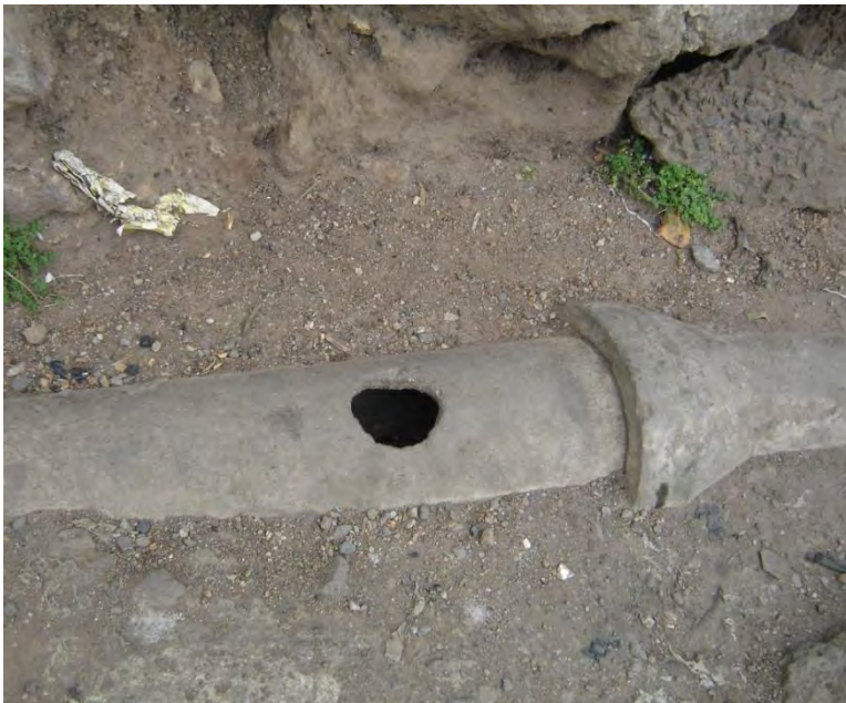
Photo 6. 2: hole dug into sewer pipe for use as a toilet. Sewage overflows at times.
