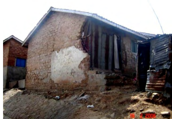
Photo 8. 19: Failing stabilised earth blocks wall in new structures Source: Author
