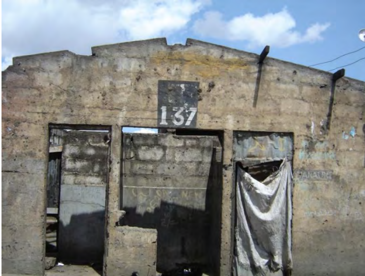
Photo 6. 1: A vandalised toilet block with a curtain on a cubicle that is still in use despite having no running water
