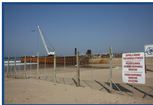
Figure 4: Battery Beach pier: one of the four officially designated piers for fishing along the Durban coastline. It is expected to be under construction until 2012 (SvG, Aug. 2010)
