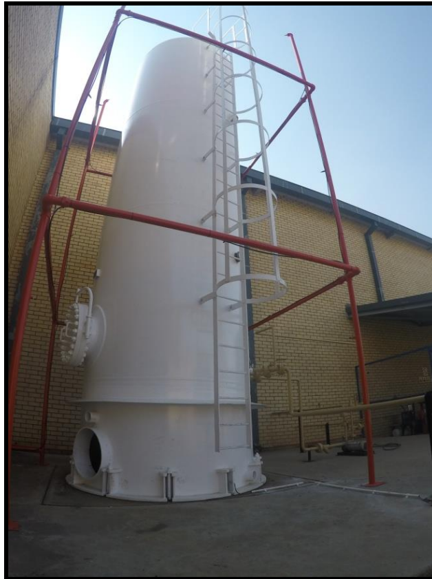
Figure 2.4 22m 3 Vertical Tank
