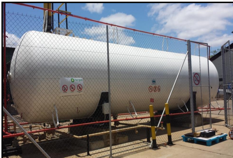
Figure 2.3 Horizontal m 3 Tank
