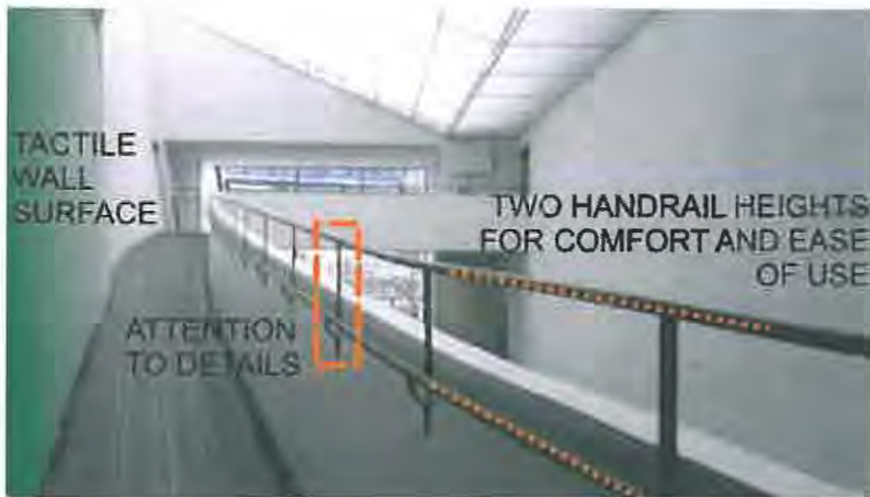
(Plate 6.16: Interior images reveal the tactile qualities of those architectural elements that connect with the human body. For example: railings, wall finish and floor finish. Source: www.kiasma.fi )
