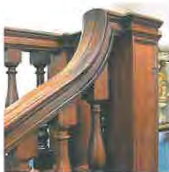
(Plate 2.6 & 2.7: The use of the sense of touch is illustrated in the difference in balustrades above.
