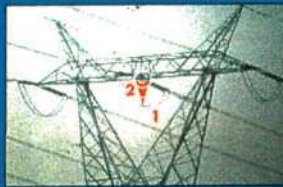
Flashover on strain tower
