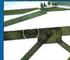
2. Bum marks on strain tower
