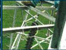
2. Bum marks on tower
