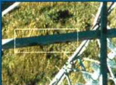
2. Bum marks on tower
