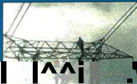
Flashover on V-srring
