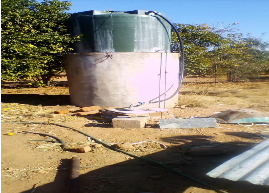
Image 4.2: The submersible pumps and storage tank
