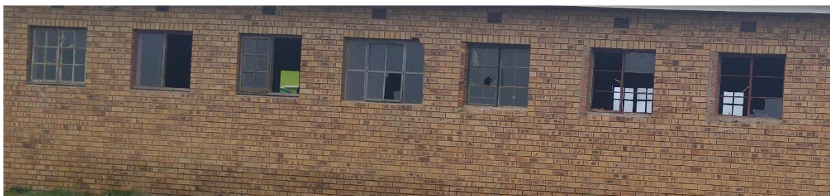
Figure 11: Picture showing a block with broken windows at Phatha Secondary School
