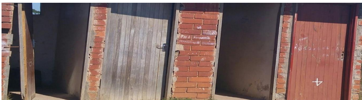
Figure 14: Picture of toilet building at Battery Secondary School showing broken doors
