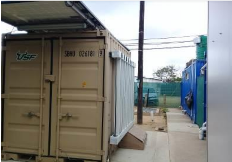
Appendix 3: Sanitation technology called NEWgenerator connected to a blue community ablution block for recovery of hydroponic nutrients, biogas and potable water.
