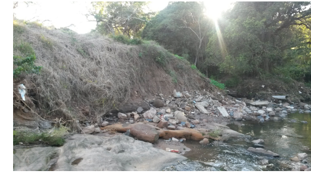
[1] - 29°49'9.2"S, 30°54'38.2"E Severe bank erosion
