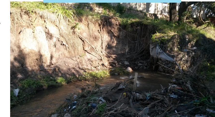
[7] - 29°48'31.9"S, 30°52'12.3"E Severe bank erosion
