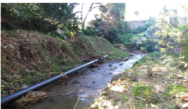
[3] - 29°48'4.8"S, 30°51'54.6"E Sewer line running along the Palmiet River
