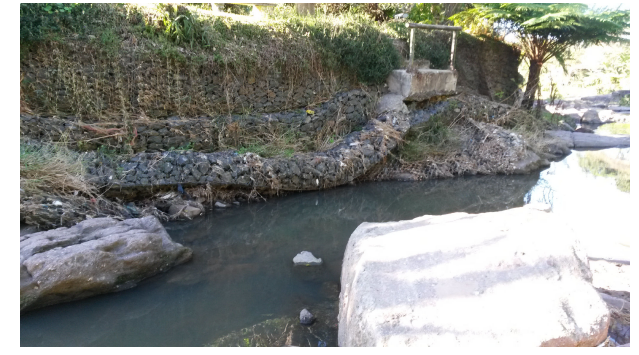
[5] - 29°49'30.6"S, 30°54'30.2"E River bank infrastructure in poor condition
