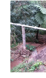
[9] - 29°48'51.8"S, 30°54'27.6"E Severe Bank Erosion along Sunnybrae Park
