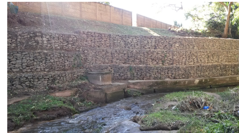
[2] - 29°48'4.6"S, 30°51'51.4"E Wall of gabion baskets implemented along the banks of the Palmiet River
