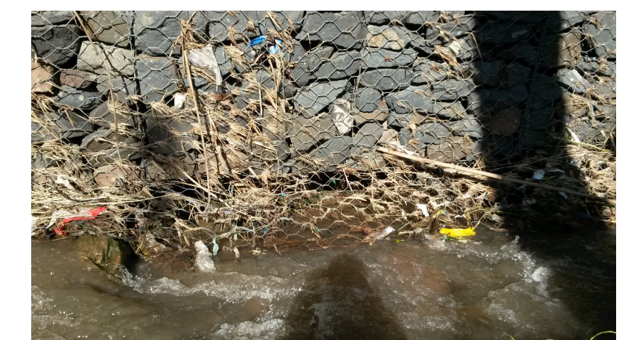
[6] - 29°48'27.7"S, 30°52'15.3"E Flow of the Palmiet River has undermined the gabion baskets
