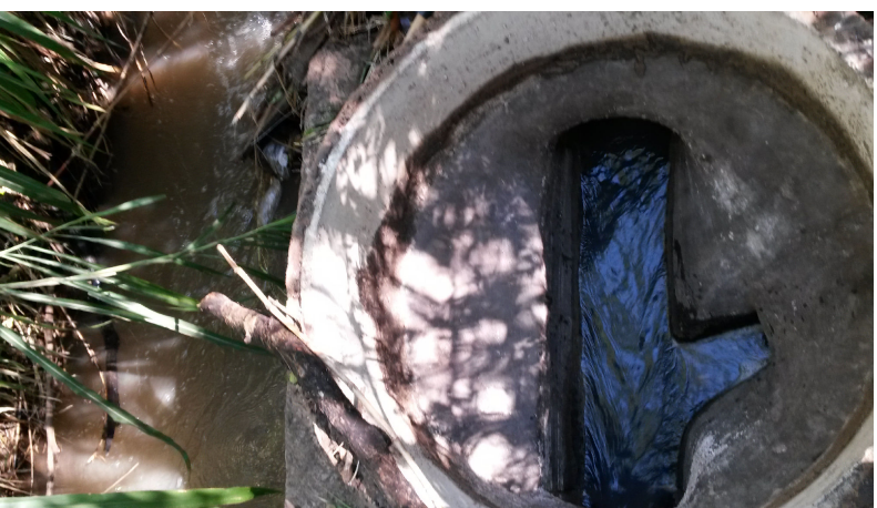
[4] - 29°48'5.6"S, 30°52'4.4"E Sewer cover missing causing potential pollution in the Palmiet River
