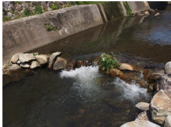
Figure 2-10: An example of a masonry drop implemented along the Akechi River in Japan (Source: Sasaki, 2016).
