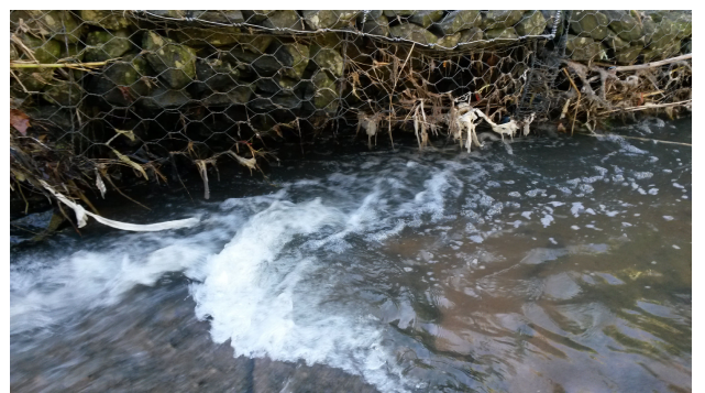
[3] - 29°49'23.0"S, 30°54'32.8"E Gabion baskets undermined
