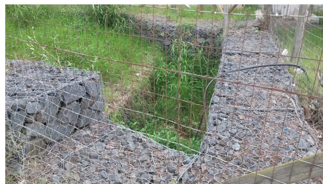
[2] - 29°48'20.5"S, 30°57'56.4"E Retention pond constructed to retain the water falling down the steep cliff.
