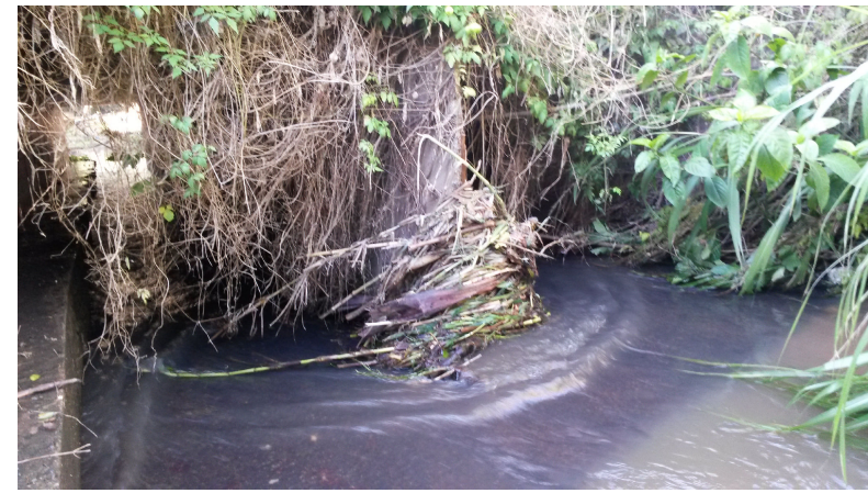
[1] - 29°48'3.73"S, 30°51'49.4"E Glenugie Road Bridge obstructing the flow of the Palmiet River
