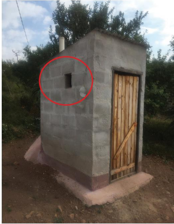
Photo 4 A 2L container hangs on the side of the toilet used for handwashing
