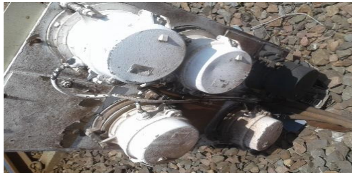
Figure 8: Vandalised robot signals
