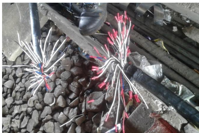
Figure 7: Cut-off copper cable
