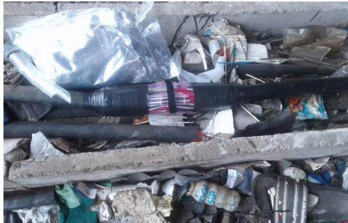
Figure 6: New instalation of stolen cable
