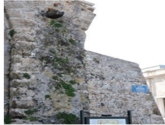
Fig. 5c. Biological Deterioration on the North Wall
