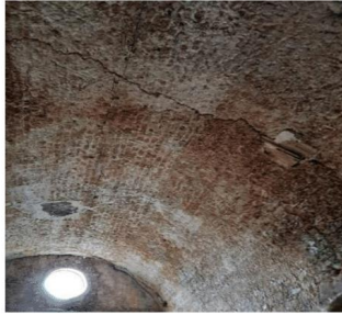
Fig. 5a. Crack on vault – inside view
