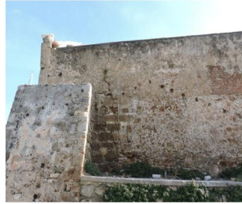
Fig. 5b. Crack on wall – West view
