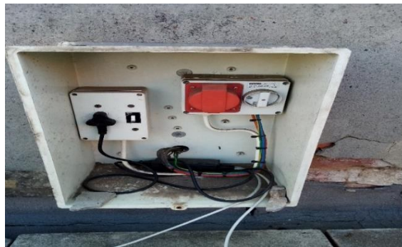
Figure 10: Transceiver Powering Box
