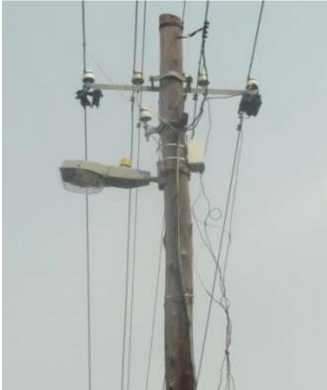
Figure 2.9: Illegal connection on a street light pole
