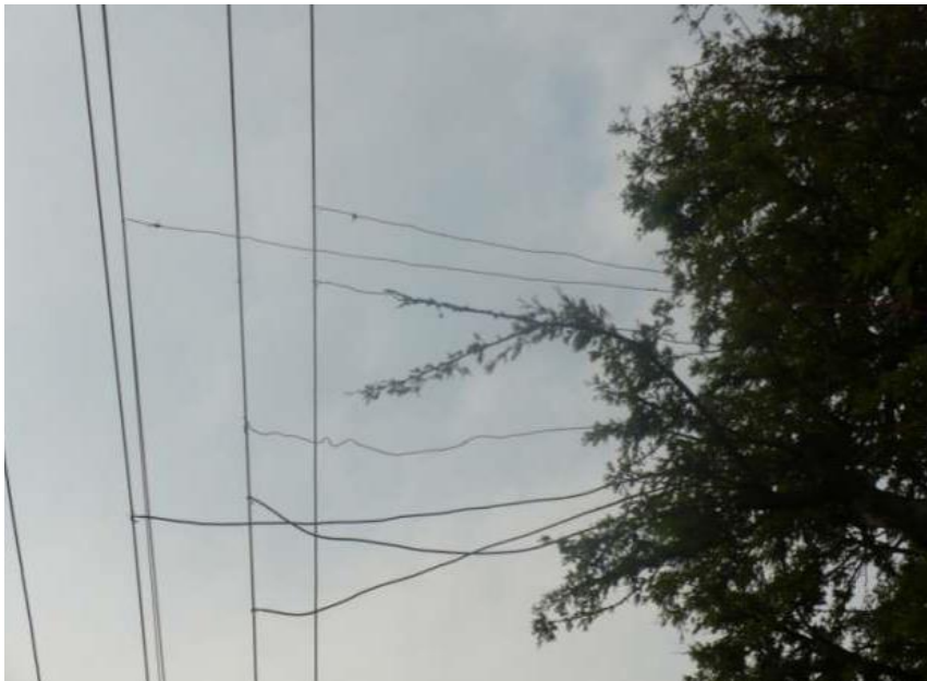
Figure 2.10: Illegal connection on the overhead line
