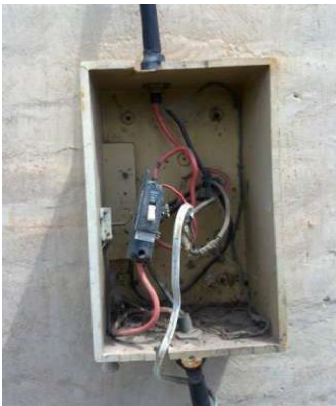
Figure 2.12: Illegal connection in meter box and ring main unit
