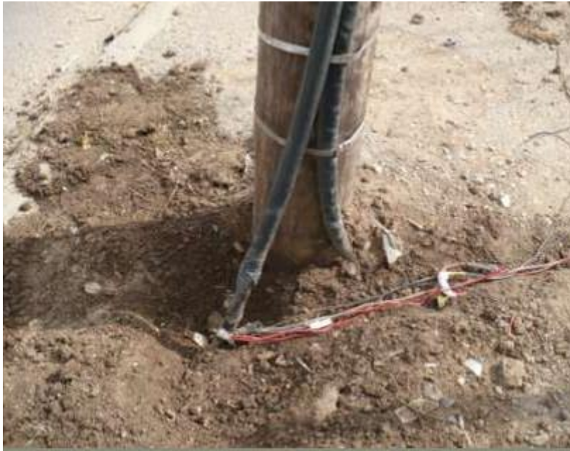
Figure 2.11: Illegal connection on the underground main line
