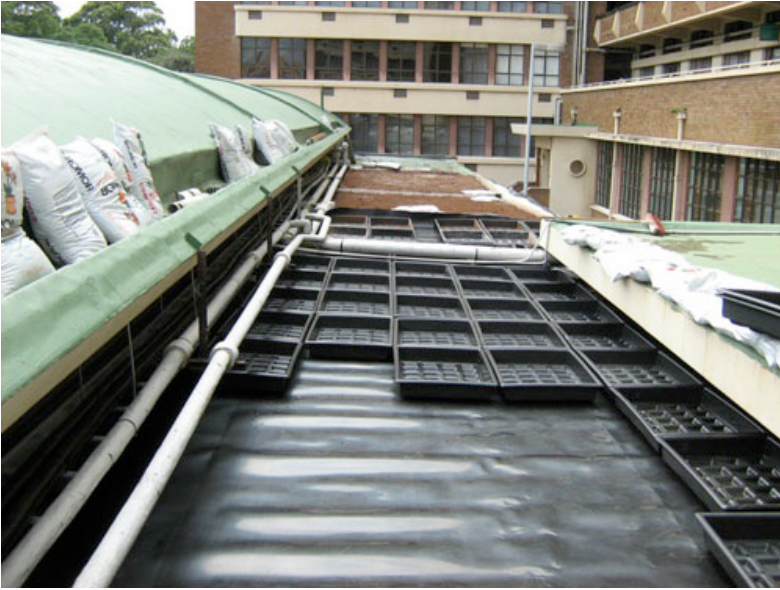
Plastic trays stacked side by side on plastic roof-sheeting underlay(waterproofing) exiting roof slab. Plates 4.3.1- Source: www.greenroofdesigns.co.za
