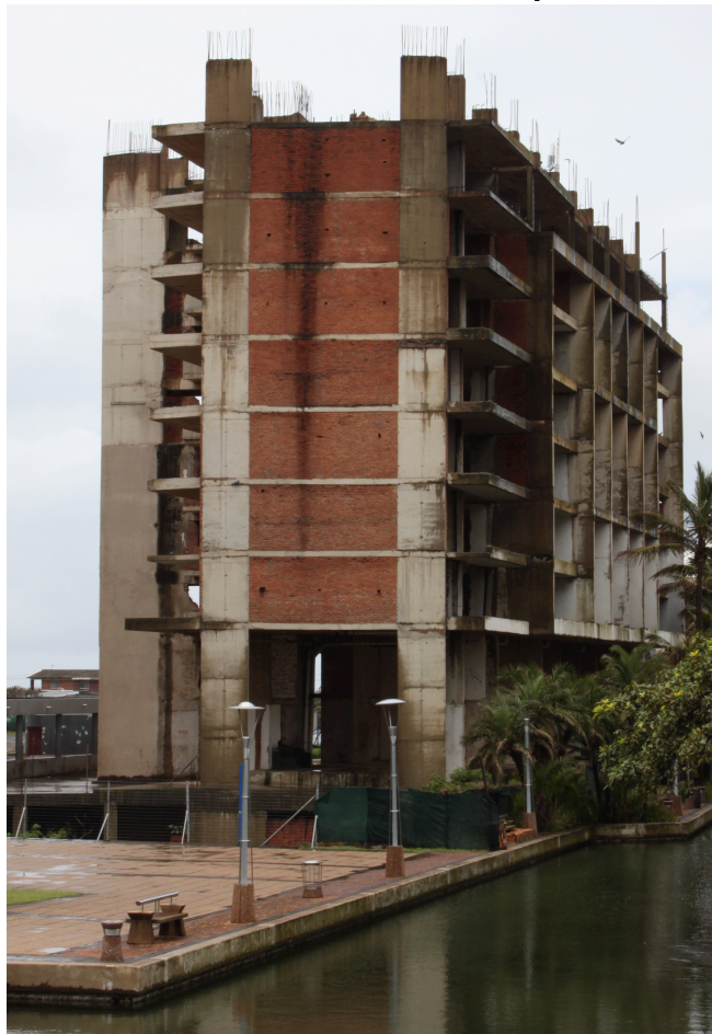
Plate 4.2.3: Image of Abandoned building at The Point Waterfront Development
