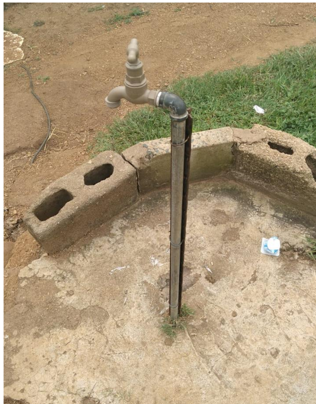
Plate 5.4. Formal tap in KwaXimba, eThekweni Municipality, KZN installed by the municipality
