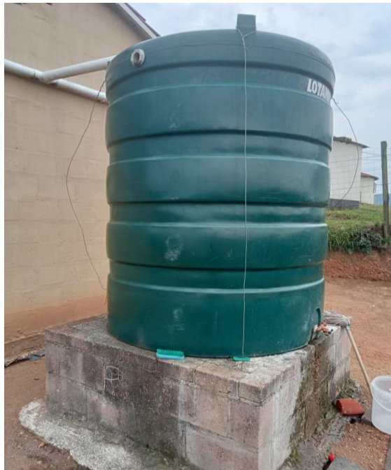
Plate 5.5. Water tank in KwaXimba, eThekweni Municipality, KZN, provided alongside the RDP
