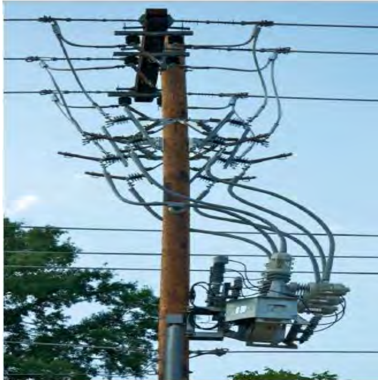
Figure 2-11: Automated Feeder Switch [60]
