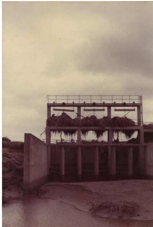
Plate (j). Cyclone Demoina damage to the Intake Works, February 1984 (Photo supplied by Nidia Brits)
