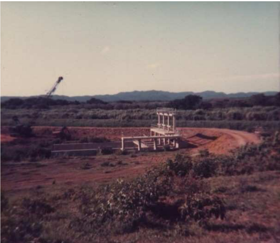
Plate (f). The almost completed intake works, 1982 (Photo supplied by Nidia Brits)
