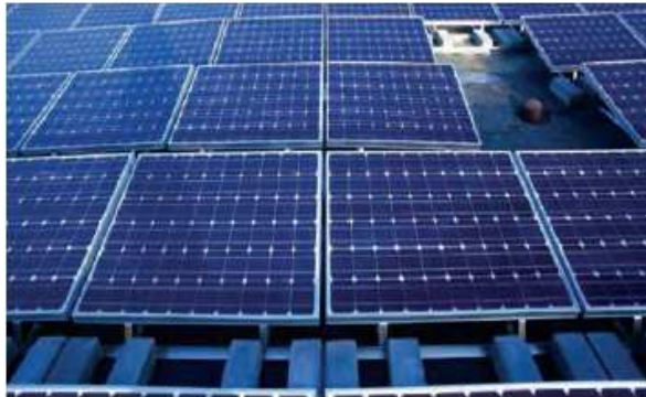
Figure 2-4 Typical PV installation [14]
