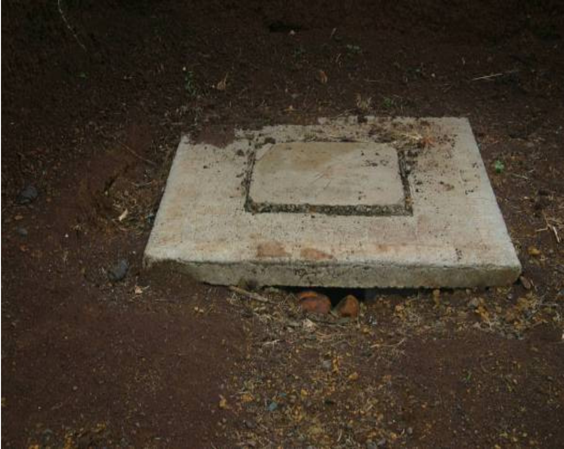
Figure 10: Infiltration area of soak-away system to facilitate effluent infiltration. The soak-away leads to a septic tank covered by a concrete slab.
