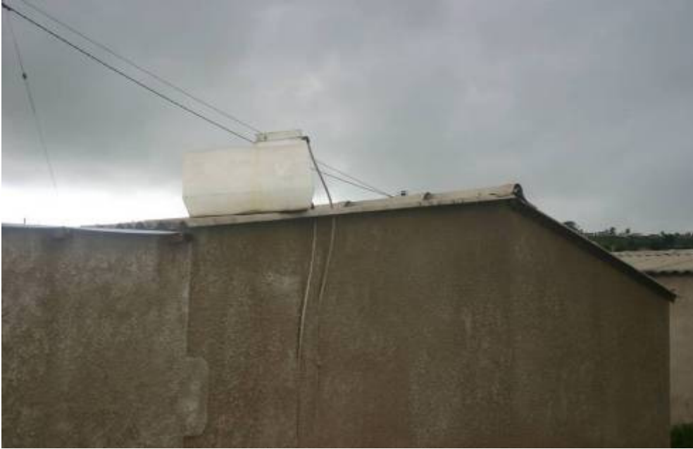
Figure 3 a: Low-pressure water tank mounted on top of the roof. (Photograph by: Siyabonga Zondi)
