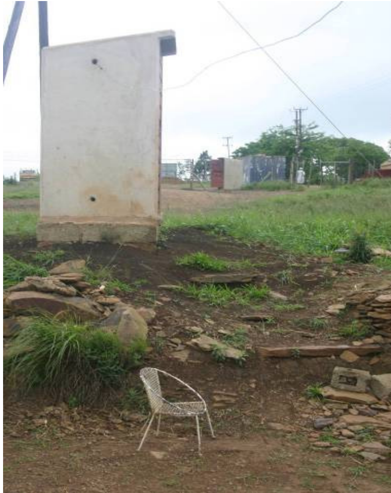
Figure 9: Poorly accessible toilet facility, particularly to disabled people. This toilet was also located very close to the public road, which may pose safety problems, especially at night. (Photograph by: Siyabonga Zondi)
