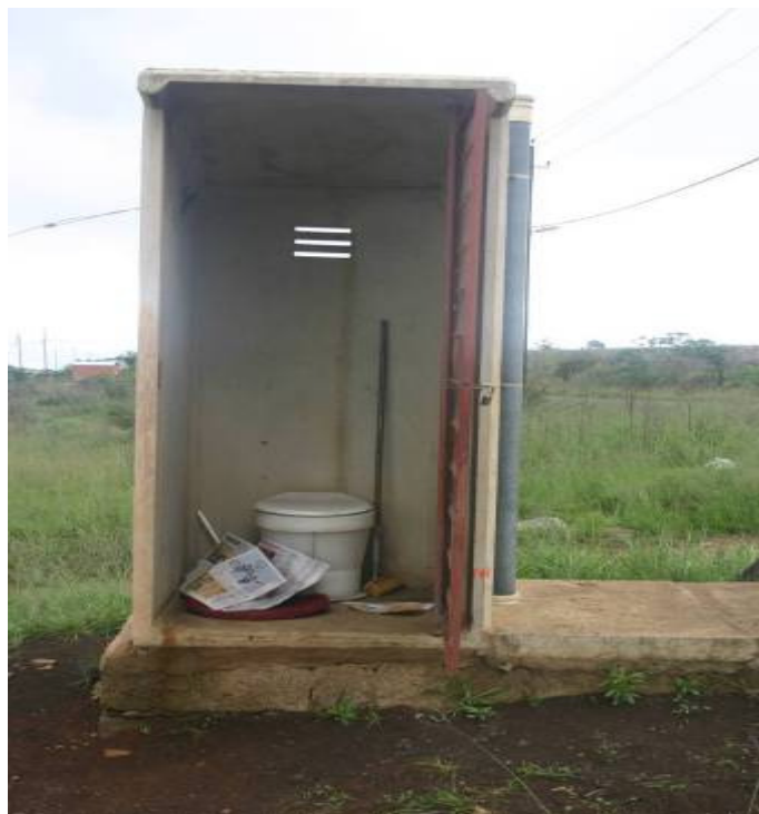
Figure 4: VIP sanitation system made of concrete slab.
