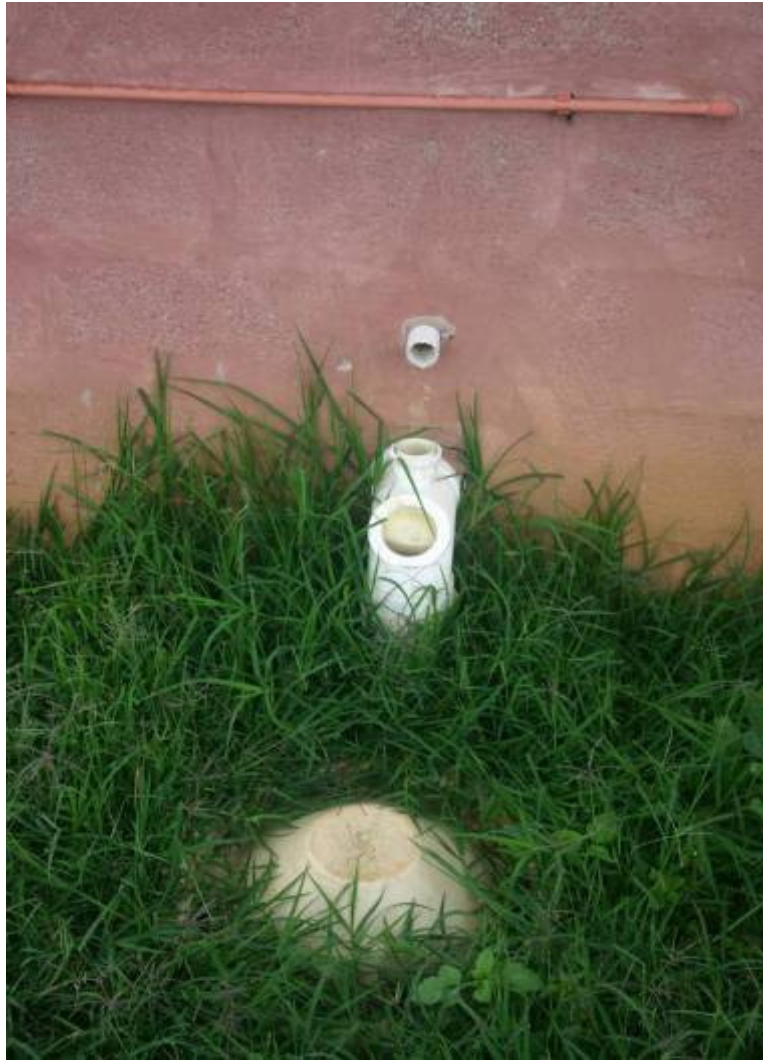
Figure 11: Element of the HS low-flush toilet system that allows for the separation of and bacteriological breakdown of faecal matter.
