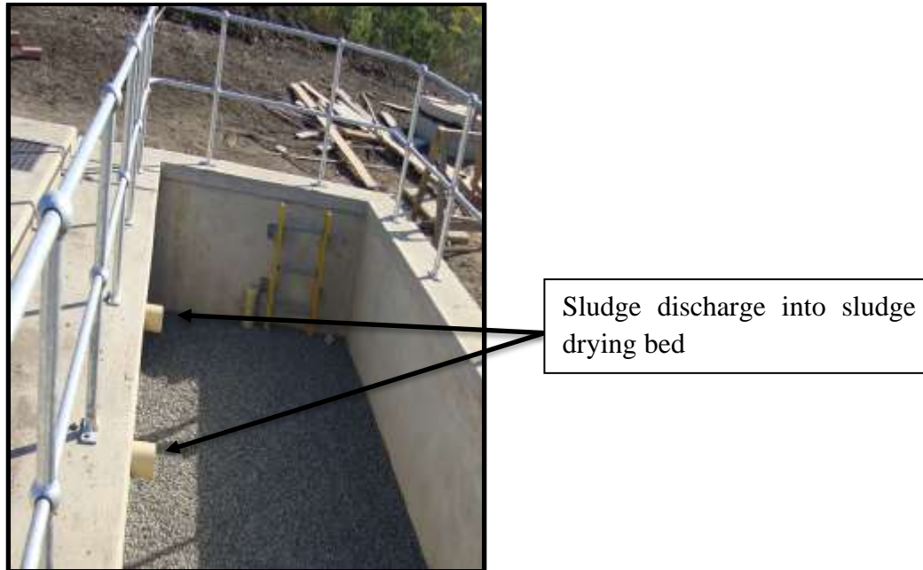
Figure 20: Sludge drying bed at NLM DEWATS showing the discharge pipes, gravel material and steel guard rails (Photo courtesy of BORDA engineers)
