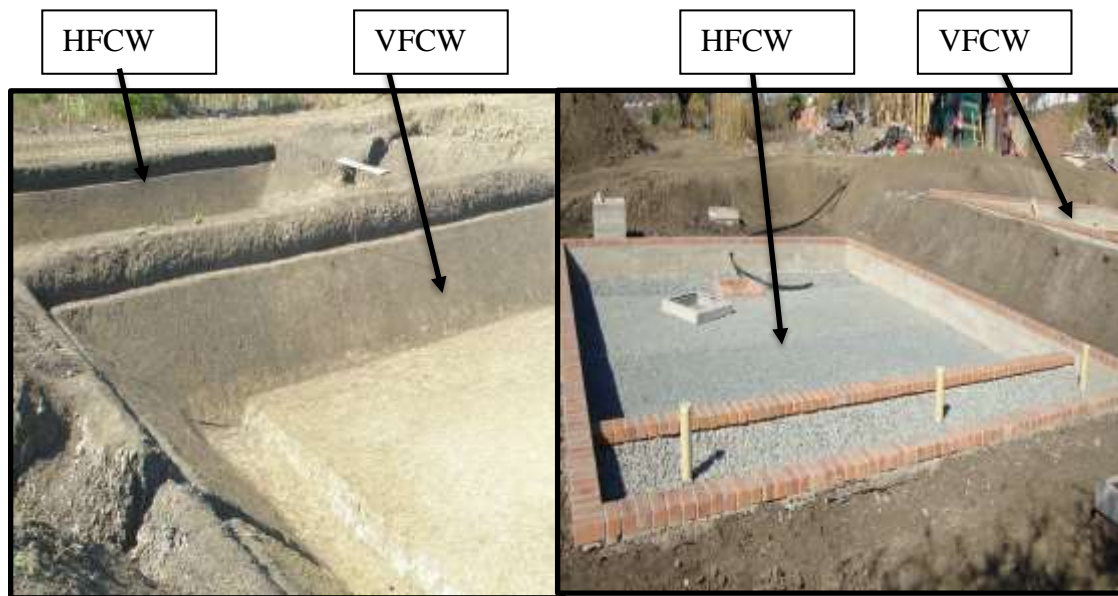
Figure 19: Left - Excavation during construction of the VFCW and HFCW showing the angled side slope at NLM DEWATS Right – Photograph showing the brick and crushed stone material used in the HFCW (Photo courtesy of BORDA engineers).
