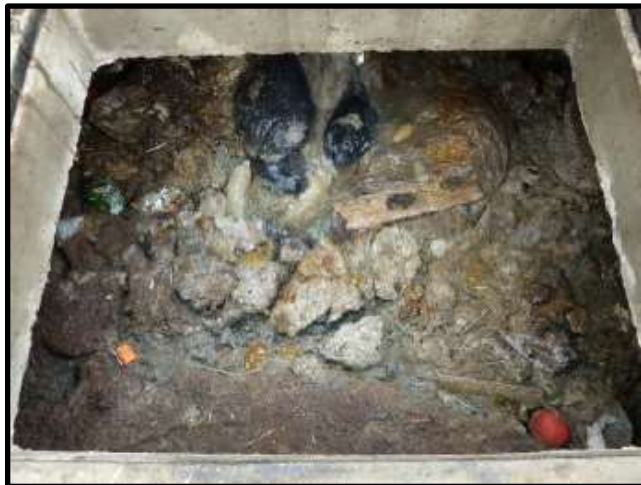
Figure 27: Foreign material accumulated inside the initial settling compartment at NLM DEWATS.
