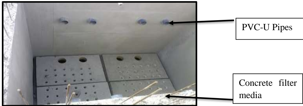
Figure 17: Photograph of a compartment of the anaerobic filter during construction showing the PVC-U pipes, perforated concrete filter media and reinforced concrete housing unit (photo courtesy of BORDA)
