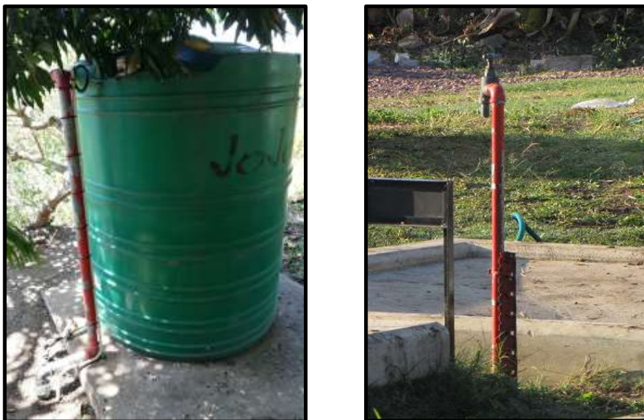
Figure 22: Right - LLDPE storage tank ("Jojo Tank") with reinforced concrete base near entrance of NLM DEWATS. Left – Standpipe at NLM that receives treated effluent from the storage tank via gravity flow.
