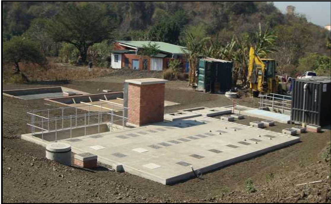
Figure 13: General overview of the NLM DEWATS site (Photo courtesy of BORDA).
