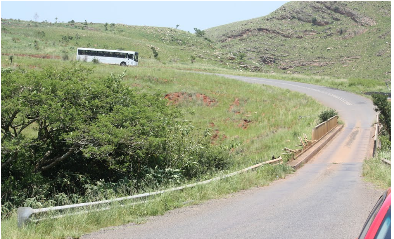
Figure 3.2: The single lane Bridge in the upper Mhlathuze River connecting the area to one of the nearest towns (source: Google Earth).
