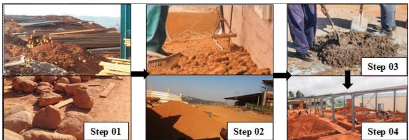
Figure 6.2f illustrates rammed earth composition process on-site, foundation and trenches construction on site. (Source: By Author, 2019).
