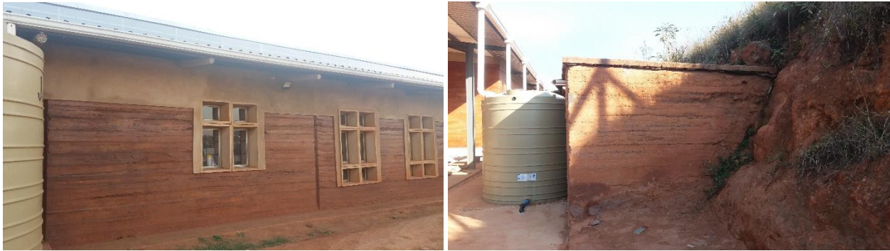
Figure 6.2h & i illustrates rammed earth wall with and without finish painting respectively. (Source: By Author, 2019).
