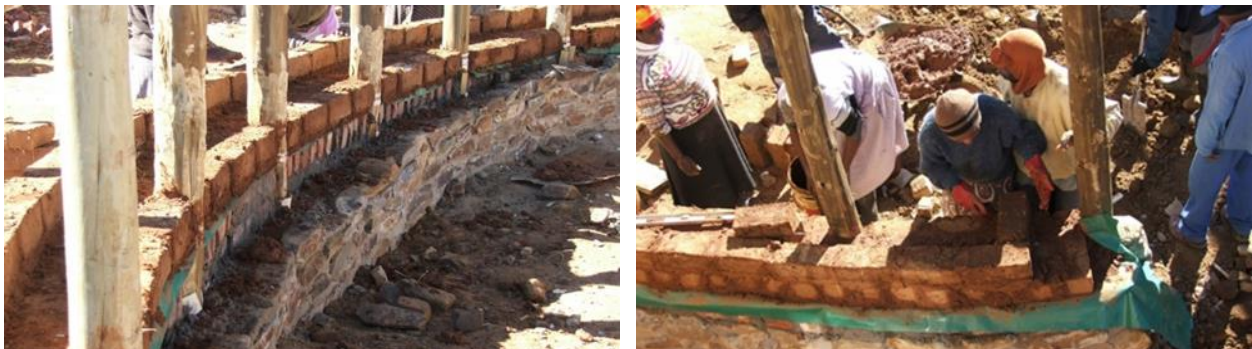
Figure 4.2b illustrating reused bricks and timber gum poles used for foundations and earth bricks used for walls as natural with good insulation materials in Seven Fountain School multipurpose building. (Source: https://www.designindaba.com/ )
