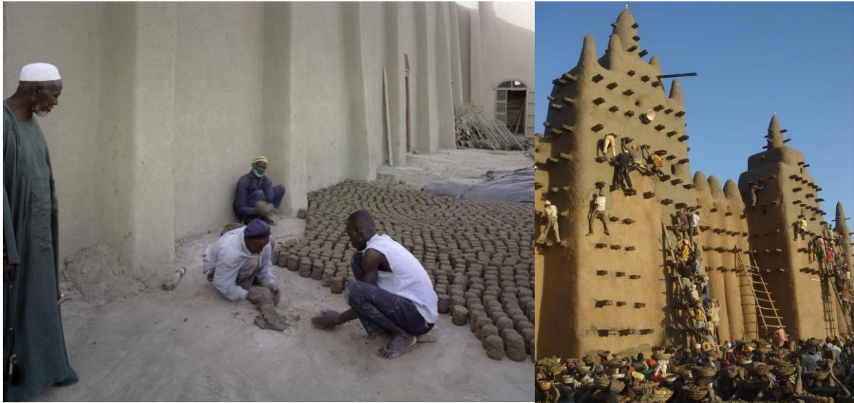
Figure 2.4c: illustrates seniors & youth engaging during construction of the Great Mosque. Figure 2.4d illustrate community participation, during renovations of Djenne Mosque in Mali. Source: https://archnet.org/sites/6395/media_contents/75605
