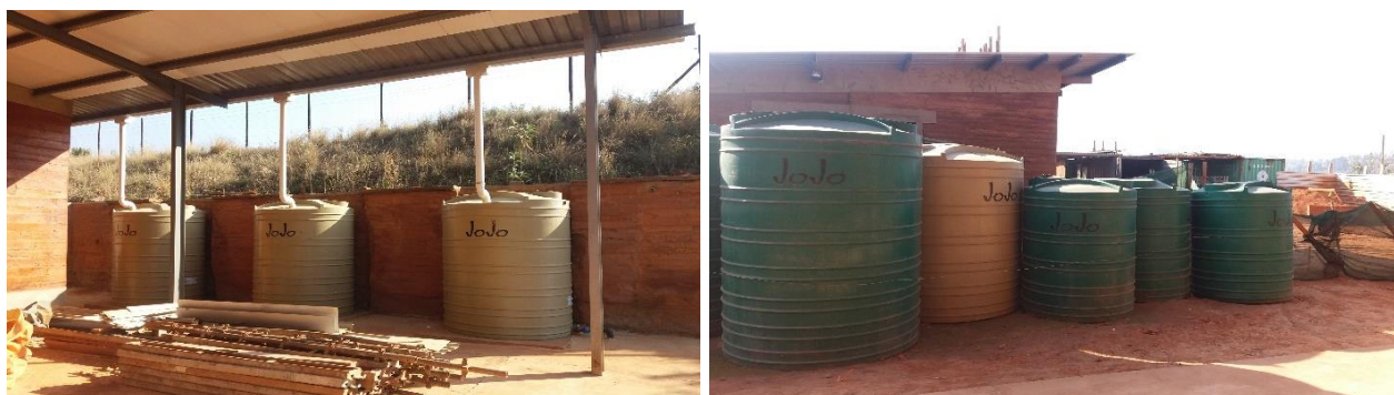
Figure 6.2n illustrates JoJo tanks collecting rainwater from the buildings and supply the entire site. (Source: By Author)
