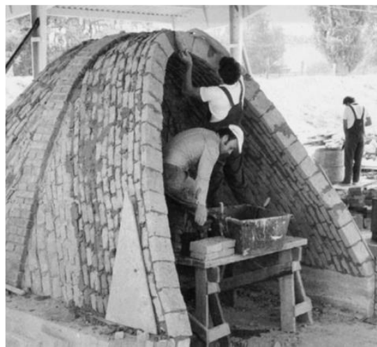
Figure 2.5k illustrate wooden moulds to make adobe blocks, and Figure 2.5l : Nubian vault made of adobe blocks under construction. The adobe can be plastered with earth plaster to achieve a smooth and attractive surface. Source: (Minke, 2006)
