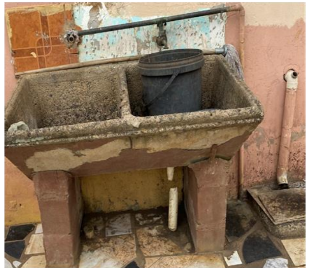
Plate 5.10 A household's dysfunctional tap with no running water within the Intaphuka community
