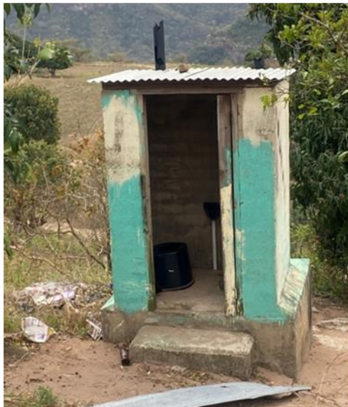
Plate 5.4 Degraded communal sanitation within the Kwazini community
