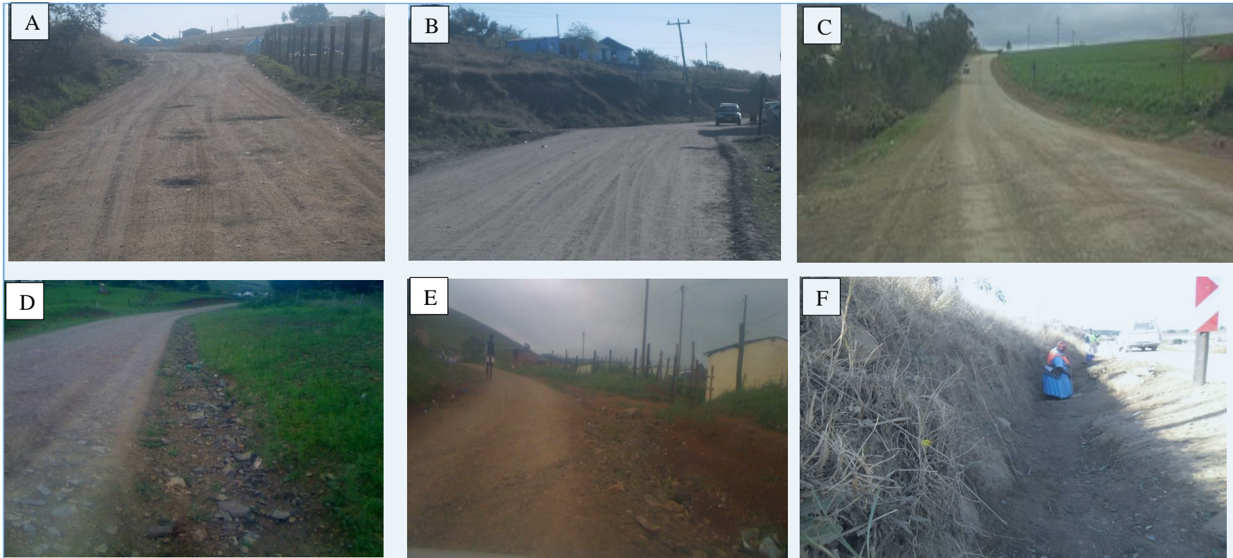
Figure 5.5: Roadside drainage conditions on some of the selected road lengths. The conditions ranged from very poor (A, B and C) to poor (D and E) and excellent (F).
