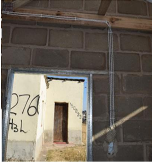
FIGURE 33. ELECTRICAL WIRES ARE PROTECTED WITH WIRE MESH AND OVER-PLASTERED (SMITH 2019)
