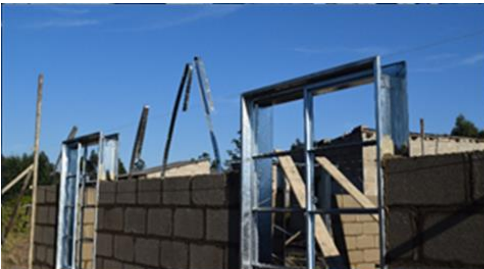
FIGURE 32. WINDOW FRAMES WITHOUT LINTELS (SMITH 2019)
