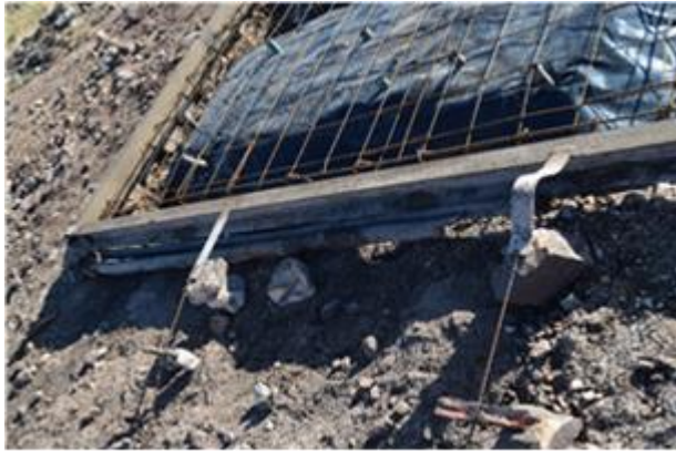
FIGURE 27. FOUNDATION METAL SHUTTER FRAME HELD IN POSITION WITH METAL STRAPS, SUPPORTED BY ROCKS (SMITH 2019)
