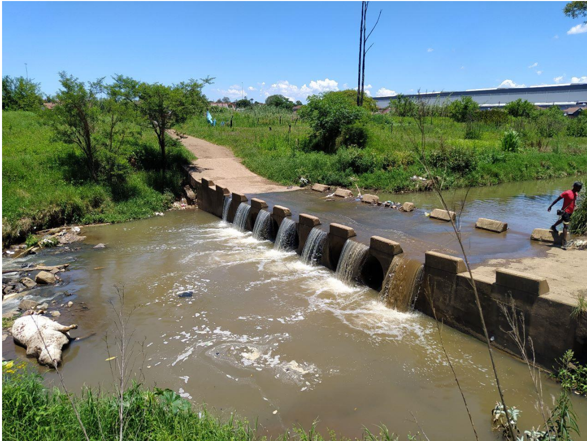
FIGURE 3.9: A poorly management culvert that was blocked during our study, showing water flowing over the culvert and not under it in Baynespruit Stream.
