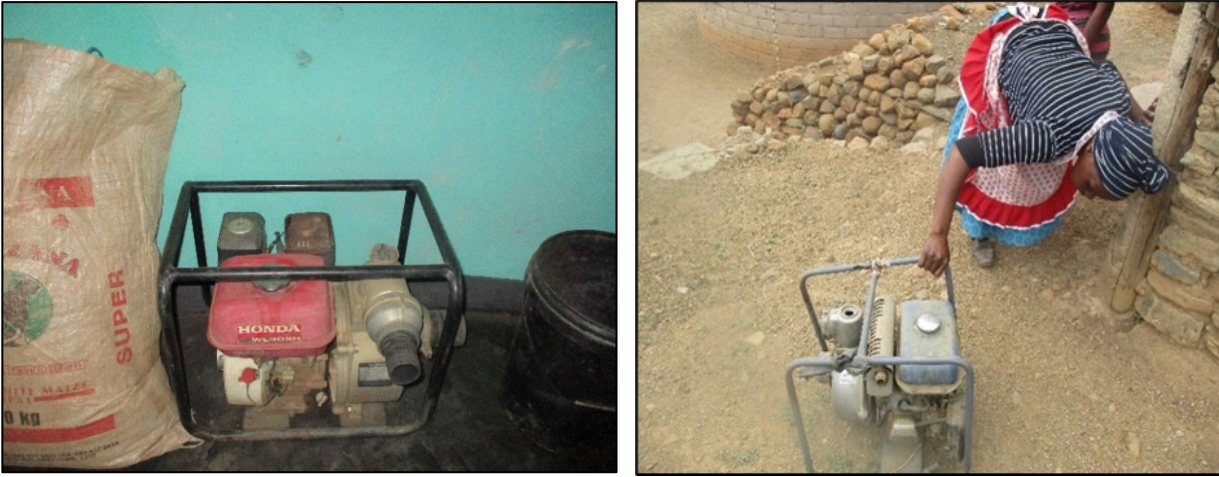
Figure 14. A pump has broken beyond repairs (left) and one that needs fixing (right) but is kept in the house until there are funds
