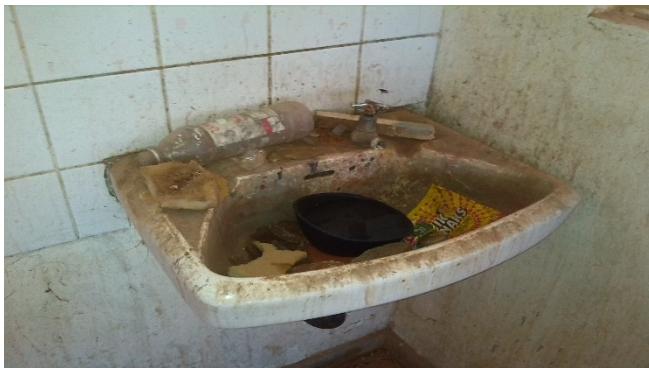
Figure 4.1: Condition of basin in the Woodwork and Carpentry workshop
