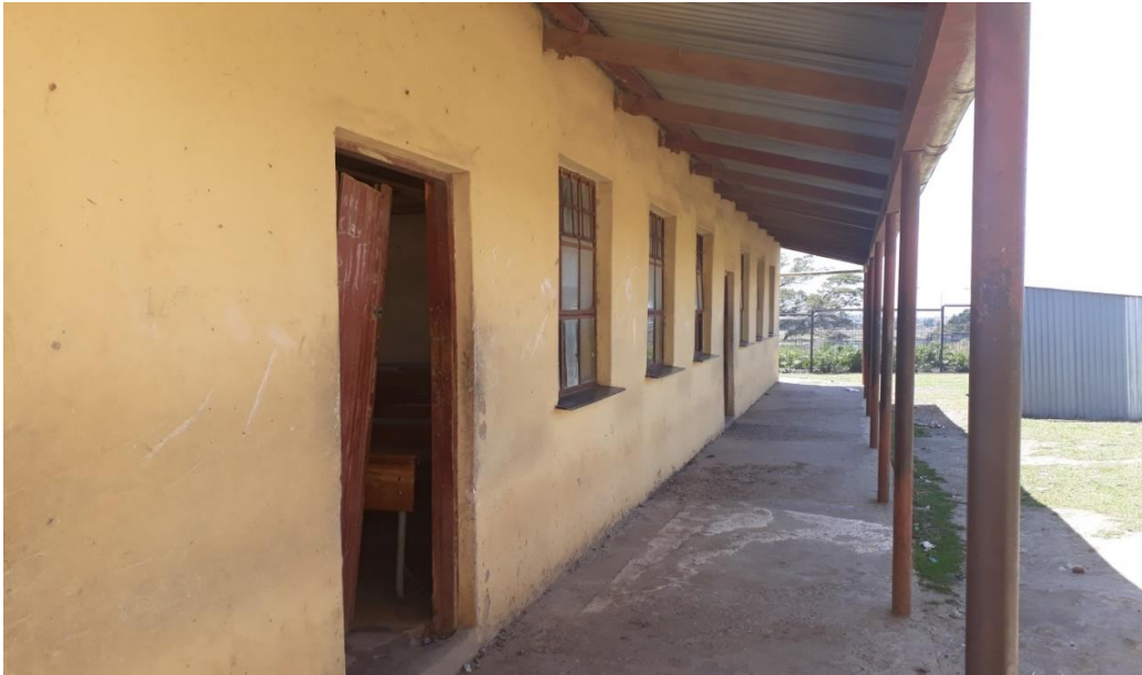
Figure 15: School C's Grade 10 block with broken doors and windows.
